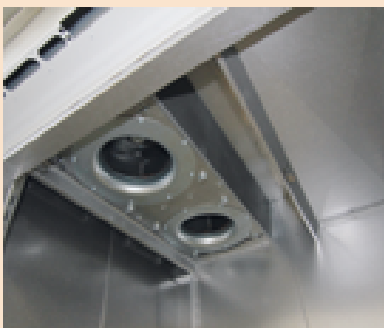
Open ceiling of the useable space with view at recirculation air fan wheels
